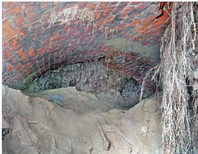
Just inside the excavated entrance a short length of lined tunnel leading to a roof fall is seen to the left.
